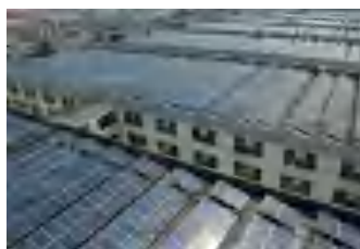
Factory roof solar photovoltaic panels
